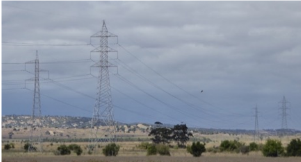
Photo: Transmission lines RMCG 1.2.2018
